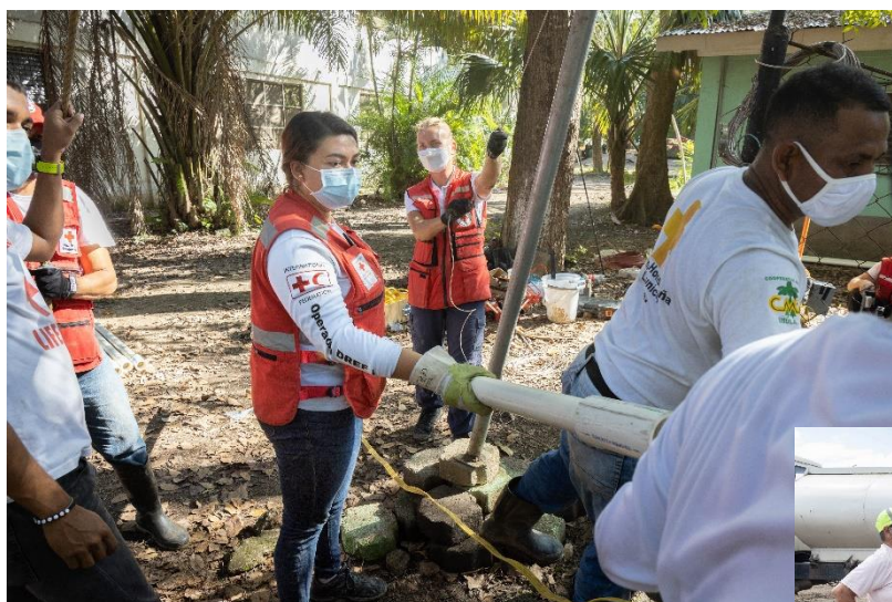
ERU team from Swedish Red Cross and Honduran Red Cross sets up water systems in San Pedro Sula after Hurricanes Eta and Iota in February 2021
